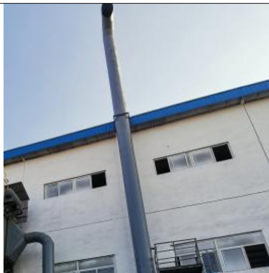
挥发窑焦粉仓上料废气排气筒
